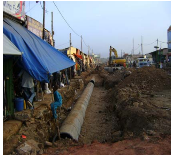
Photo 12: Ongoing drainage works and road construction activities in the business centre part of Jimma town.
